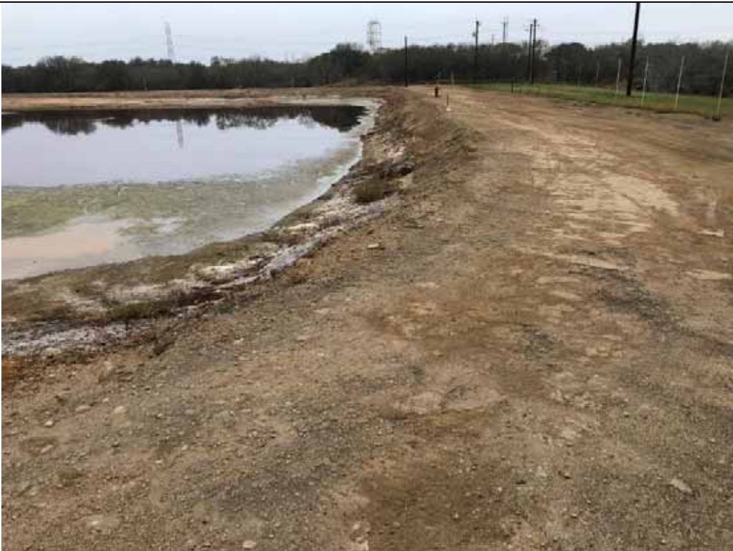
Photograph: 14 Evaporation Pond – standing on the northeast corner – facing west. Photo taken 12/14/2021.
