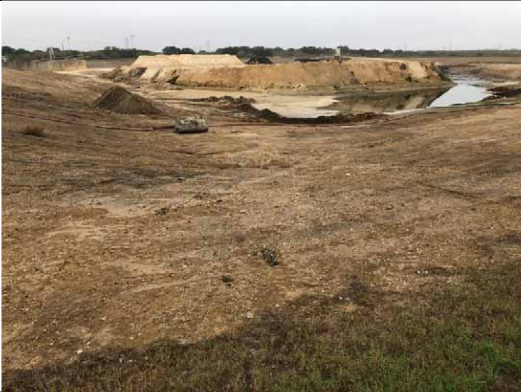
Photograph: 7 Fly Ash Landfill – standing on southeast corner – facing west. Radial stacker located in southwest corner and stormwater discharge piping in southeast corner of landfill. Photo taken 12/14/2021.
