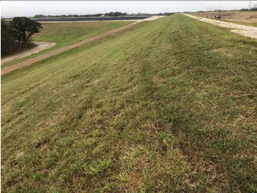
Photograph: 6 Fly Ash Landfill – standing on northeast corner – facing south. Photo taken 12/14/2021.
