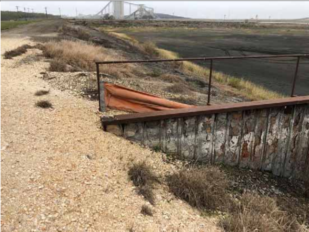
Photograph: 22 North Bottom Ash Pond – standing on northeast corner – facing south. Photo taken 12/14/2021.
