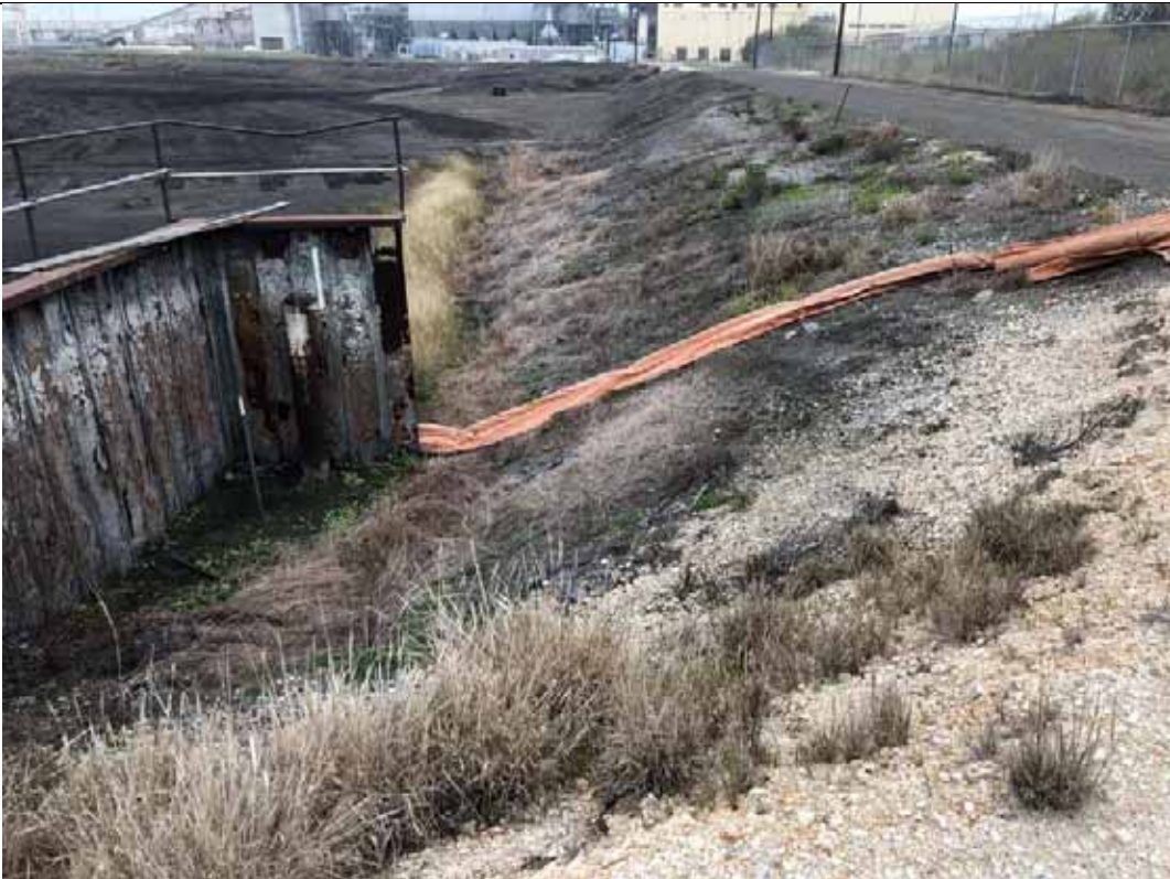
Photograph: 21 North Bottom Ash Pond – standing on northeast corner – facing west. Photo taken 12/14/2021.
