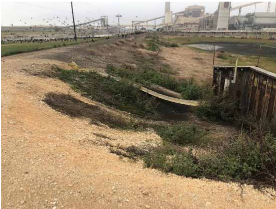
Photograph: 30 South Bottom Ash Pond – standing on southeast corner – facing west. Photo taken 12/14/2021.
