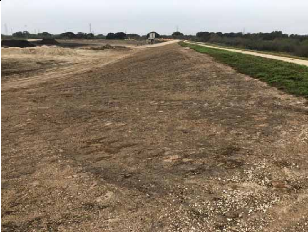
Photograph: 3 Fly Ash Landfill – standing on northwest corner – facing south. Photo taken 12/14/2021.
