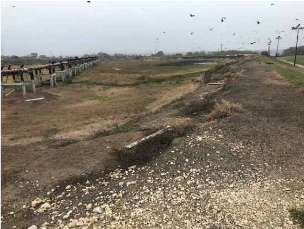
Photograph: 32 South Bottom Ash Pond – standing on southwest corner – facing east. Photo taken 12/14/2021.
