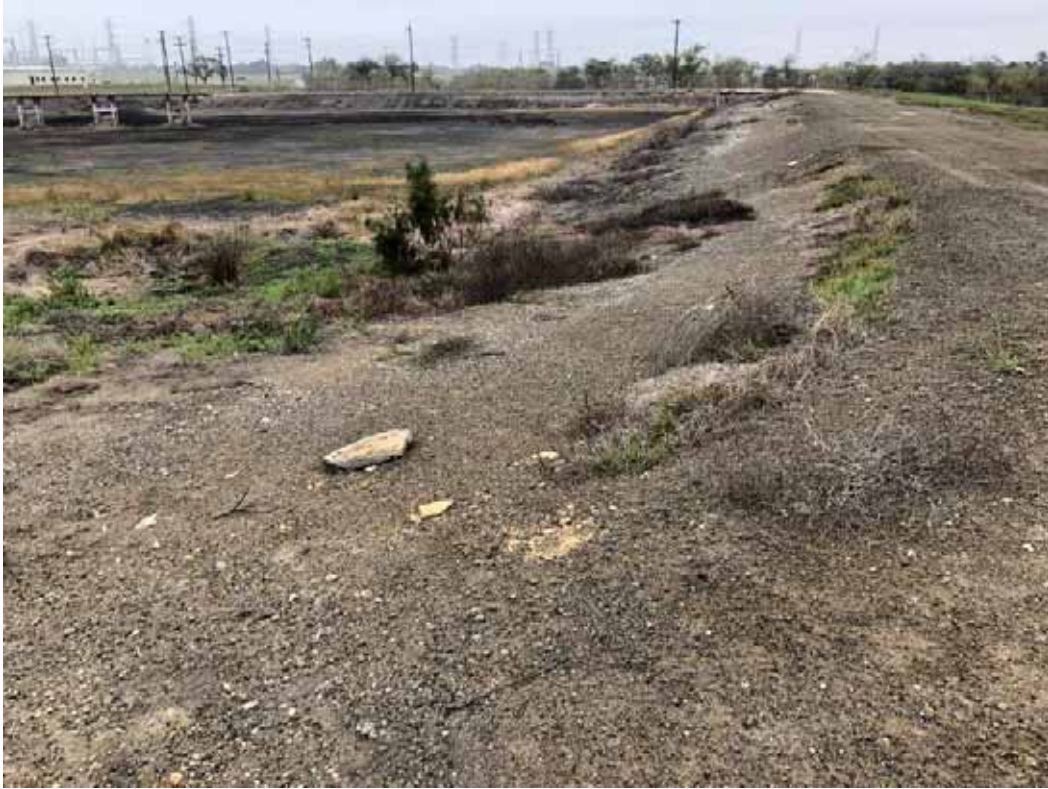
Photograph: 23 North Bottom Ash Pond – standing on southeast corner – facing north. Photo taken 12/14/2021.
