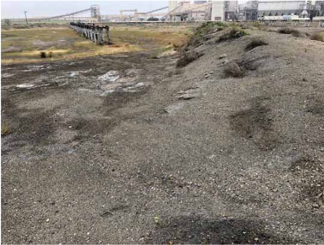
Photograph: 25 South Bottom Ash Pond – standing on northeast corner – facing west. Photo taken 12/14/2021.
