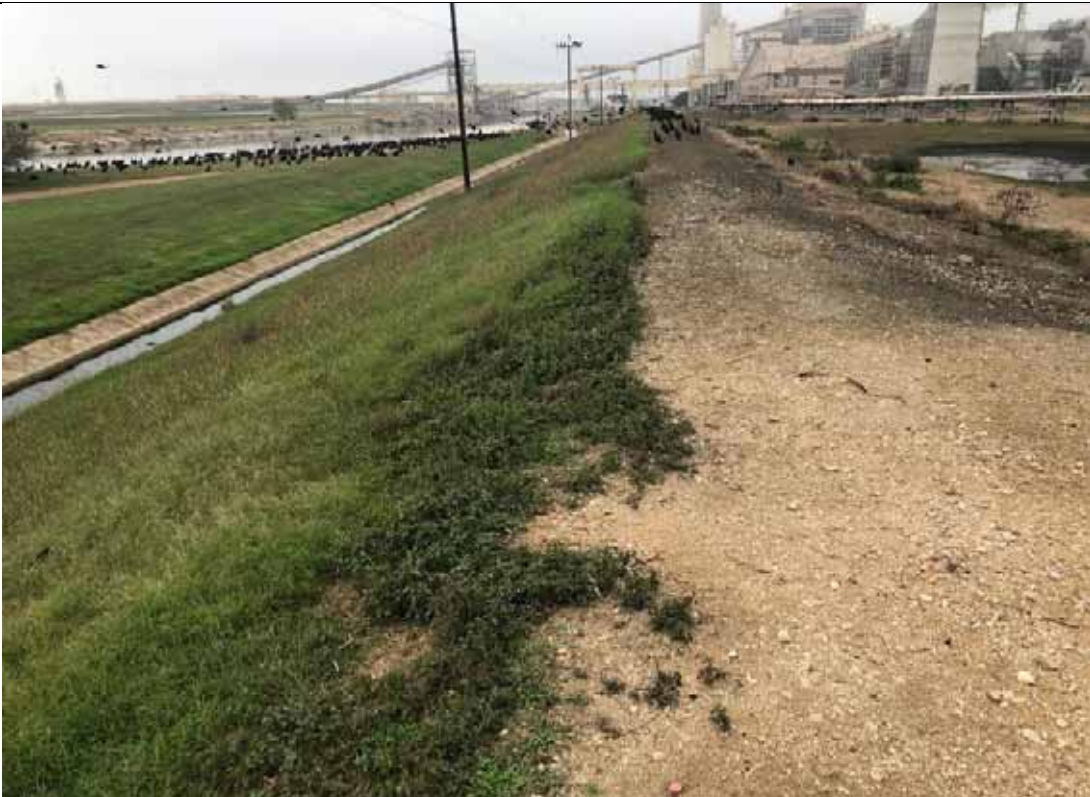
Photograph: 31 South Bottom Ash Pond – standing on southeast corner – facing west. Photo taken 12/14/2021.
