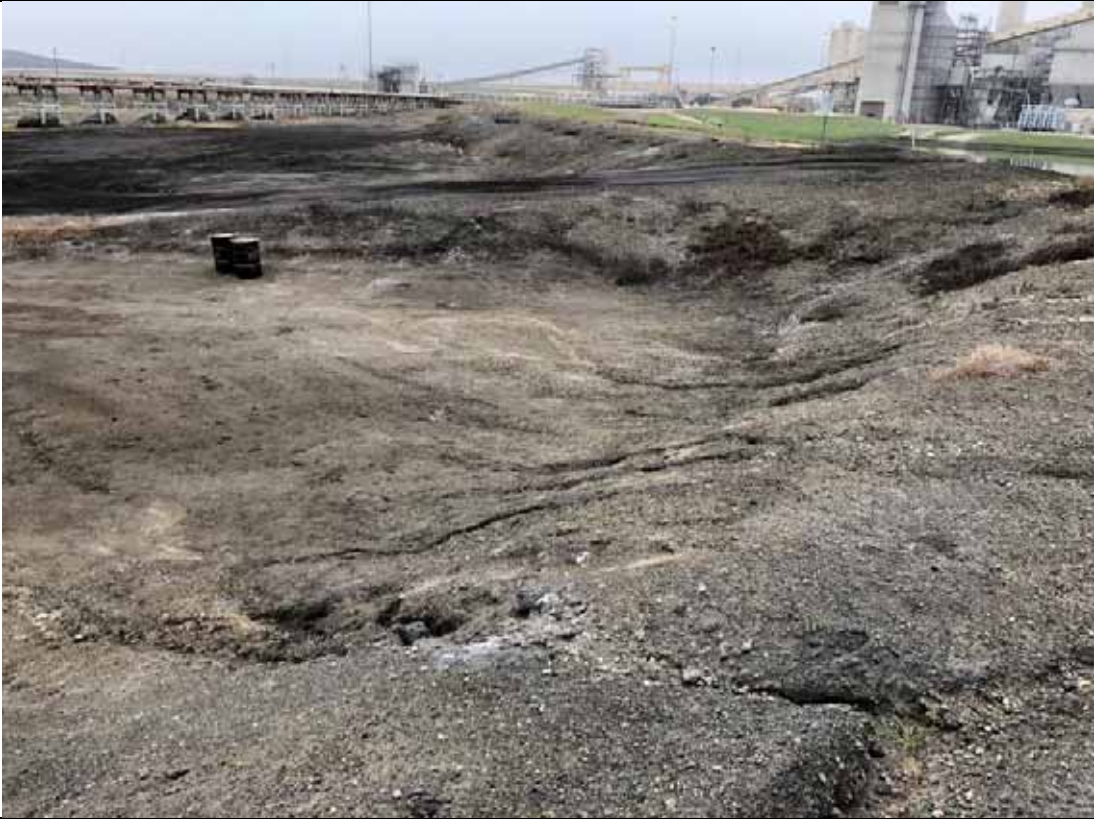
Photograph: 17 North Bottom Ash Pond – standing on northwest corner – facing southwest. Photo taken 12/14/2021.
