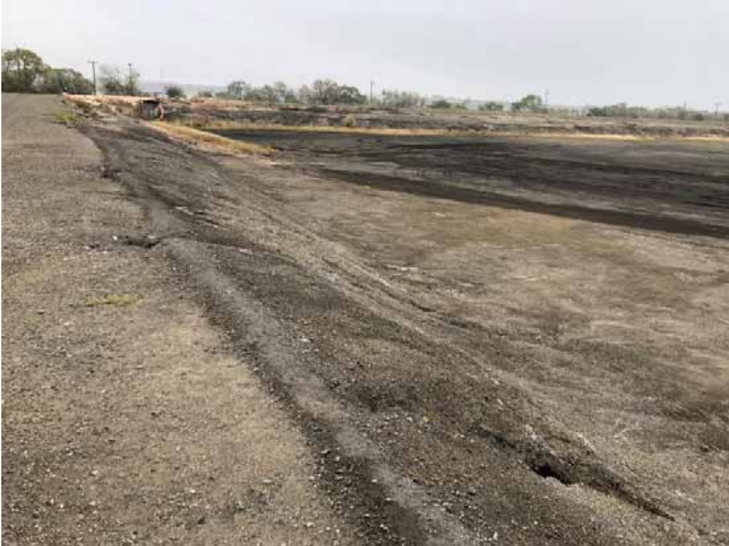
Photograph: 18 North Bottom Ash Pond – standing on northwest corner – facing east. Photo taken 12/14/2021.
