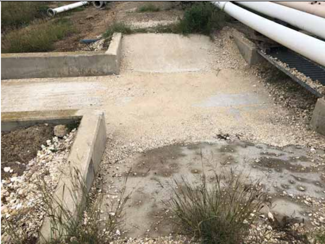
Photograph: 36 South SRH Pond – standing on the east berm – spillway structure. Photo taken 12/14/2021.
