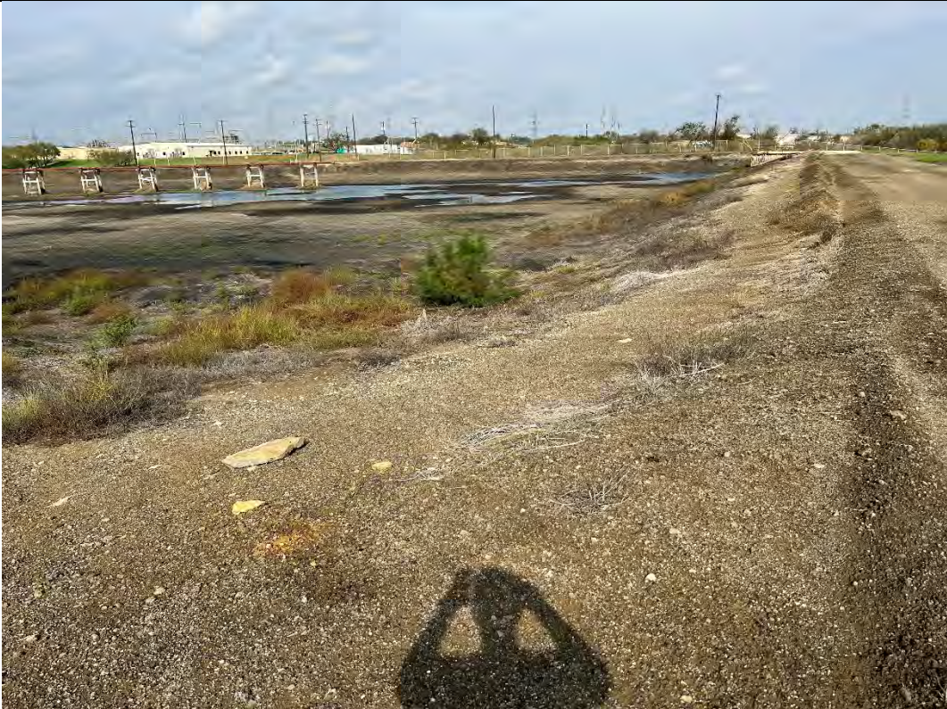
Photograph: 23 | North Bottom Ash Pond – standing on southeast corner – facing north. Photo taken 12/13/2022.
