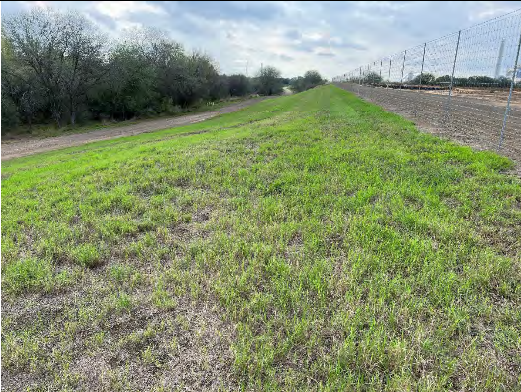
Photograph: 12 Evaporation Pond – standing on the northeast corner – facing south. Photo taken 12/13/2022.
