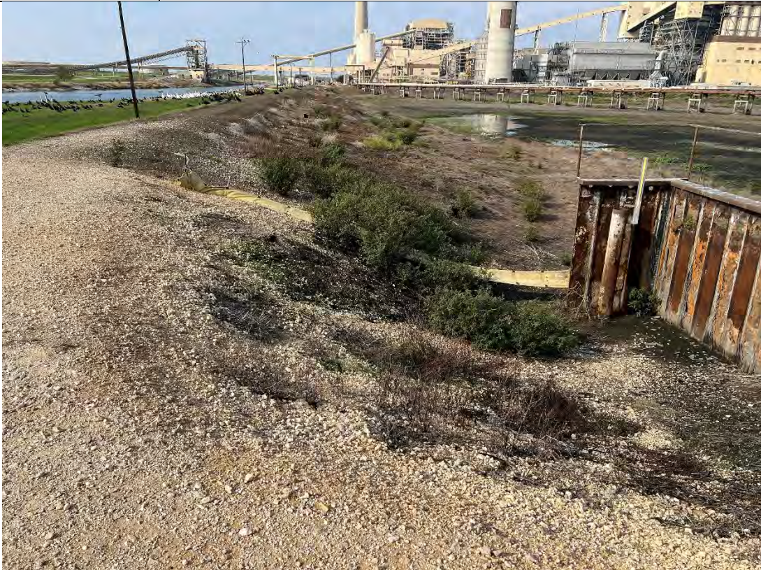
Photograph: 30 | South Bottom Ash Pond – standing on southeast corner – facing west. Photo taken 12/13/2022.
