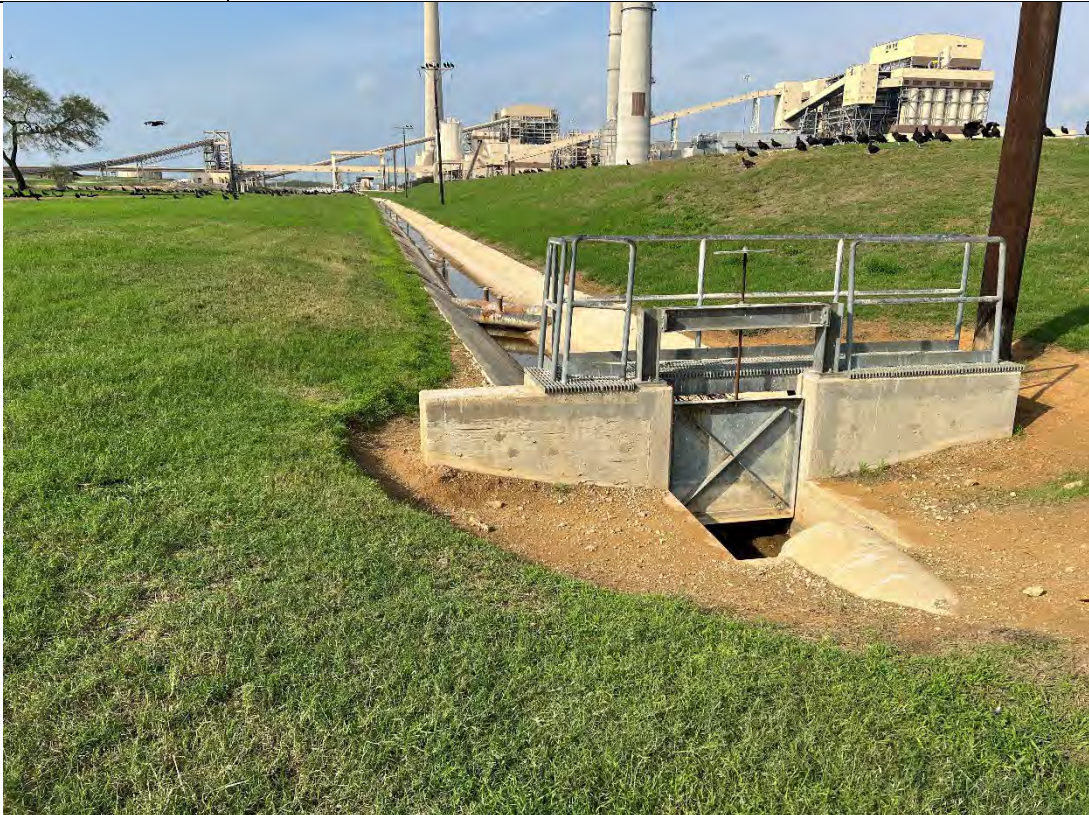
Photograph: 28 South Bottom Ash Pond – standing on southeast corner – facing west. Photo taken 12/13/2022.
