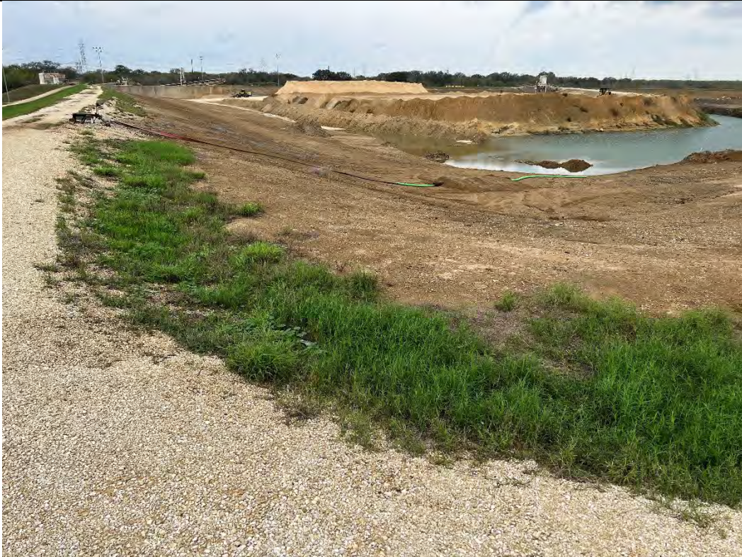
Photograph: 7 Fly Ash Landfill – standing on southeast corner – facing west. Radial stacker located in southwest corner and stormwater discharge piping in southeast corner of landfill. Photo taken 12/13/2022.
