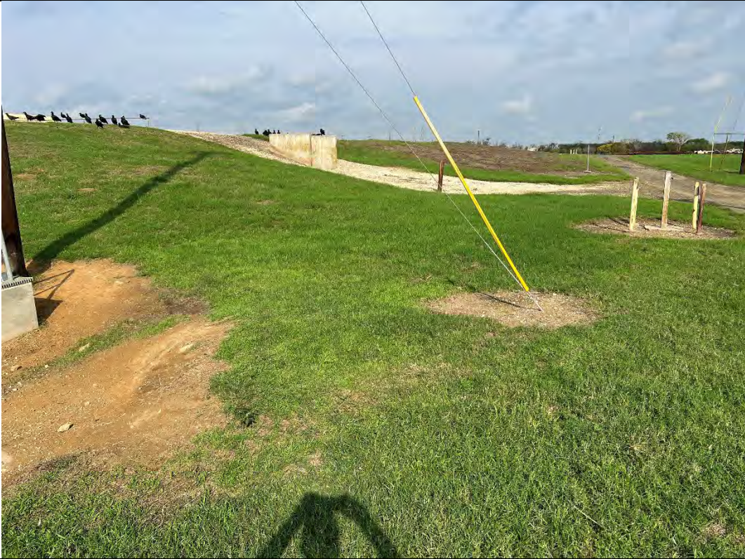
Photograph: 27 South Bottom Ash Pond – standing on southeast corner – facing north. Photo taken 12/13/2022.
