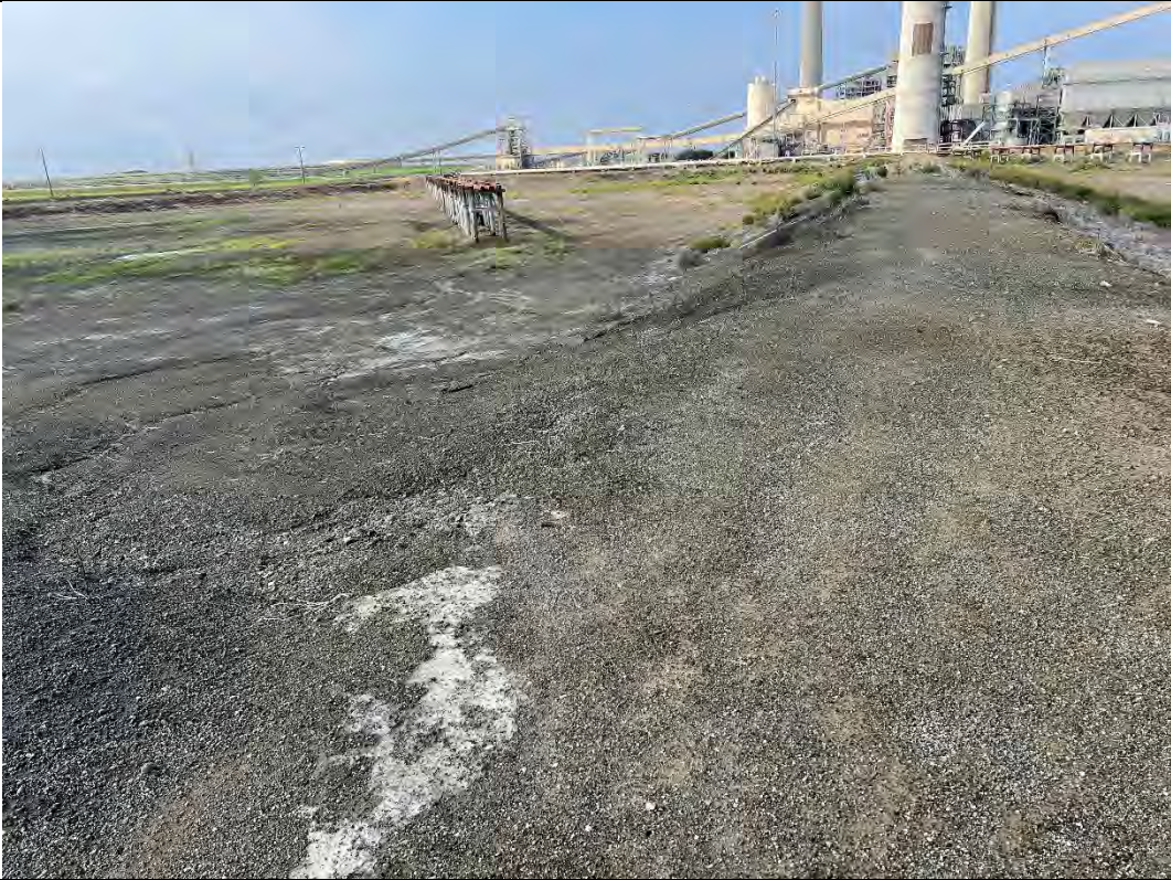
Photograph: 25 South Bottom Ash Pond – standing on northeast corner – facing west. Photo taken 12/13/2022.
