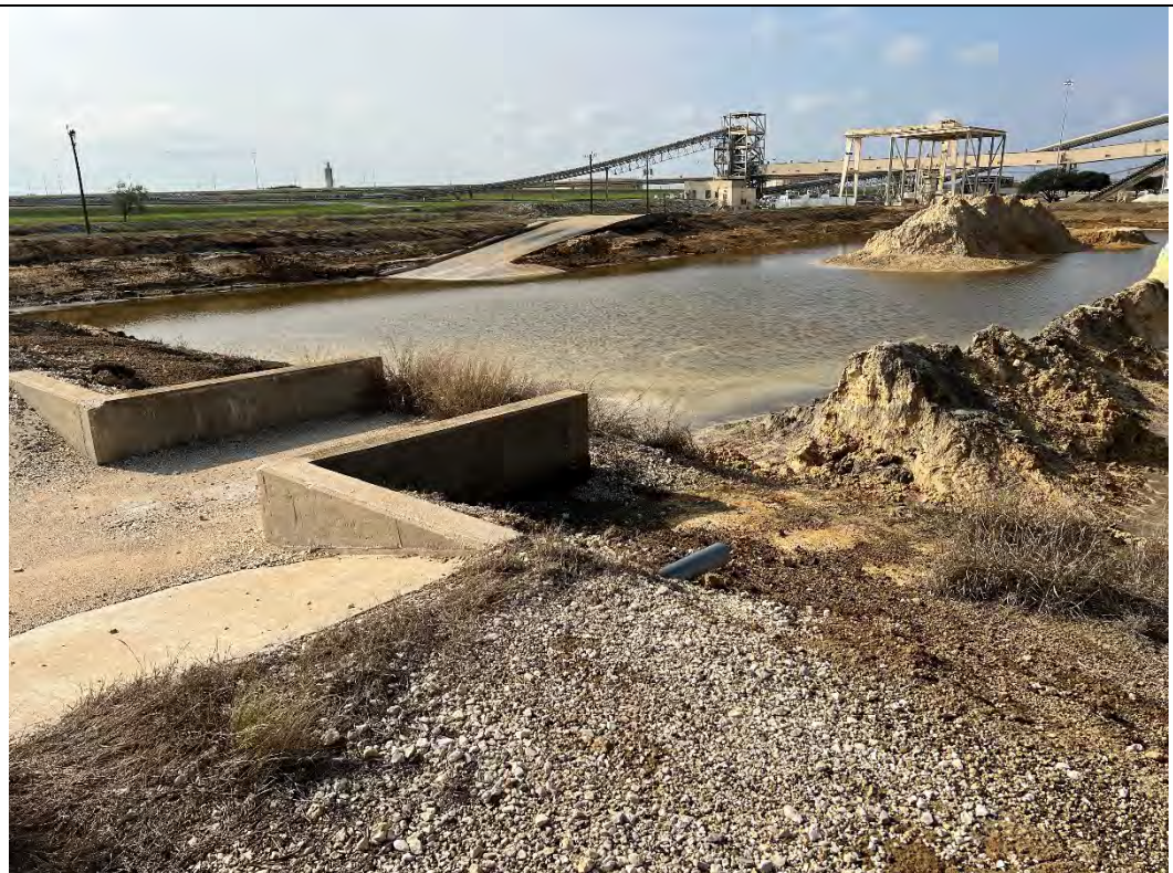
Photograph: 34 South SRH Pond – standing on the northeast corner facing southwest – spillway structure. Photo taken 12/13/2022.
