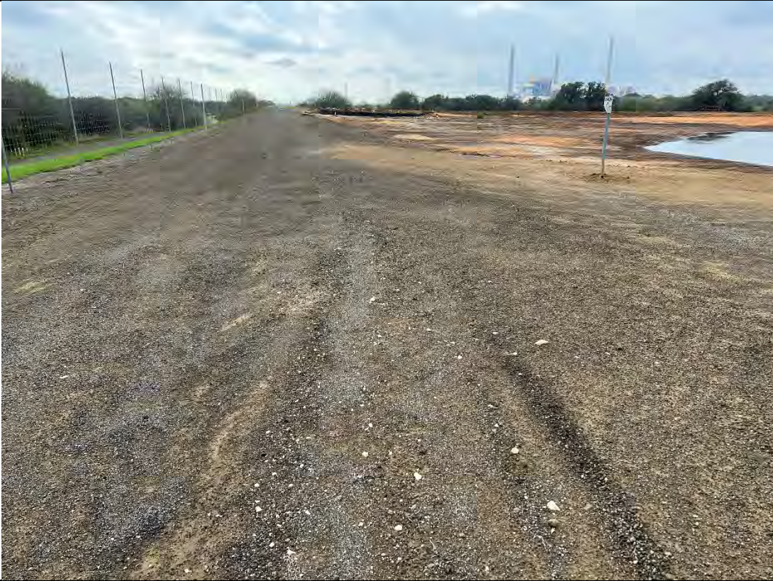
Photograph: 13 Evaporation Pond – standing on the northeast corner – facing south. Photo taken 12/13/2022.
