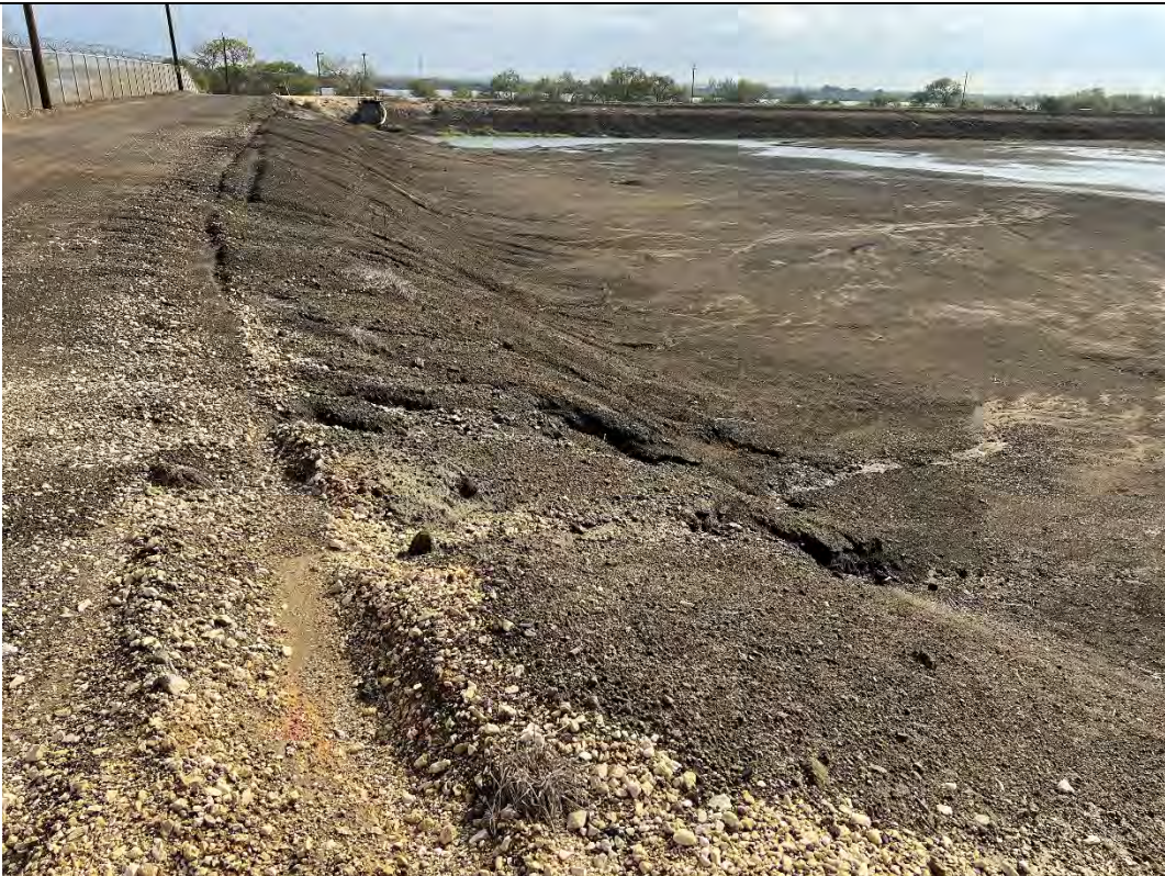
Photograph: 18 North Bottom Ash Pond – standing on northwest corner – facing east. Photo taken 12/13/2022.
