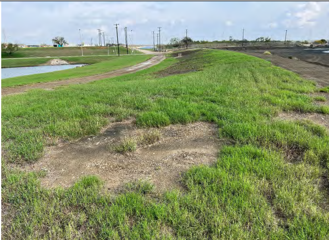
Photograph: 20 North Bottom Ash Pond – standing on southwest corner – facing northeast. Photo taken 12/13/2022.
