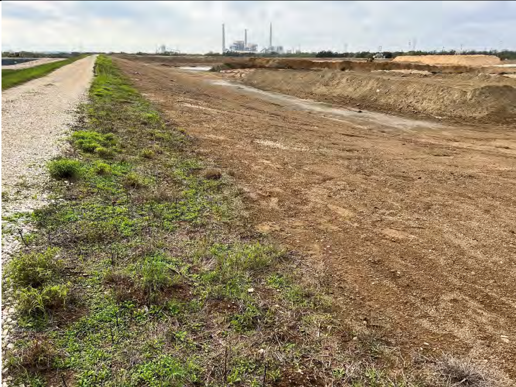
Photograph: 5 Fly Ash Landfill – standing on northeast corner – facing south. Photo taken 12/13/2022.
