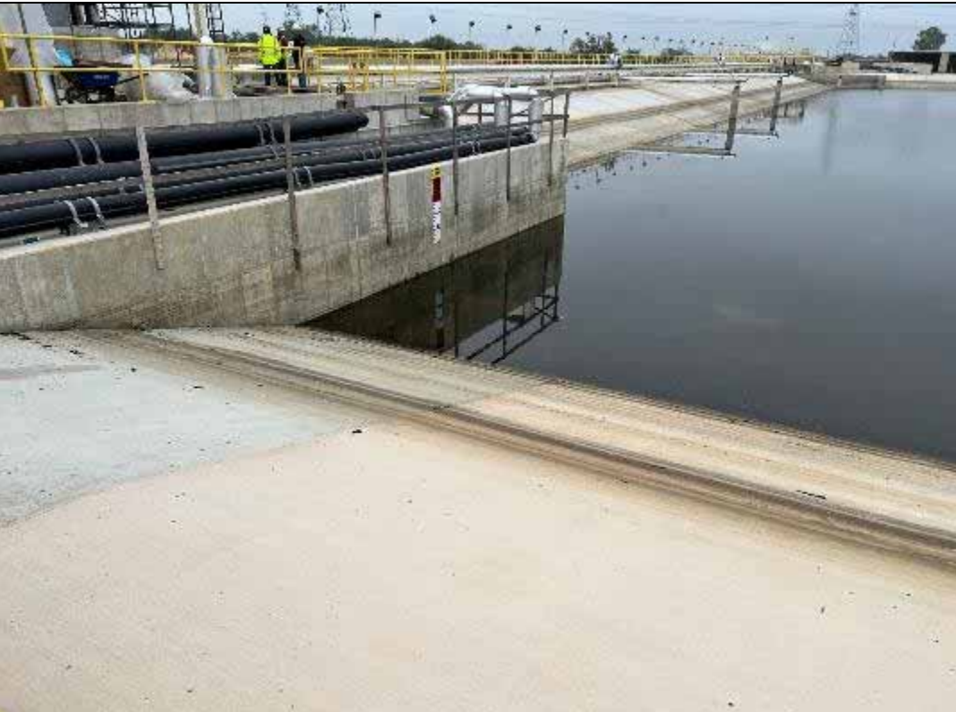
Photograph: 62 East Plant Drains Pond – standing on the southwest corner – facing north. Photo taken 11/16/2023.
