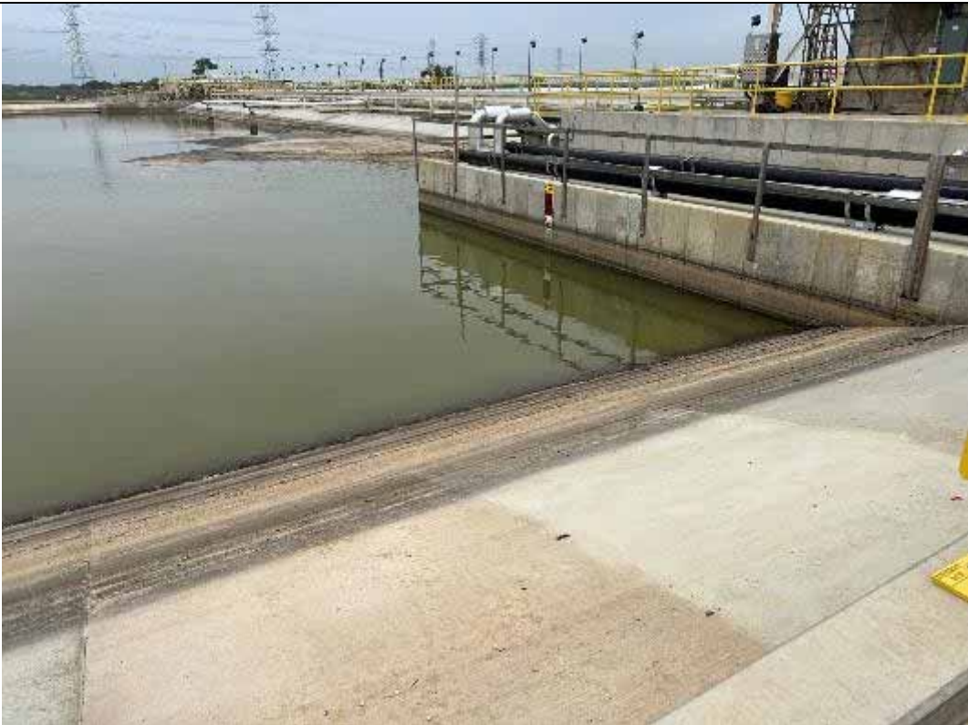
Photograph: 50 West Plant Drains Pond – standing on the southeast corner – facing north. Photo taken 11/16/2023.
