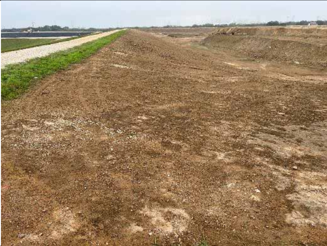
Photograph: 5 Fly Ash Landfill – standing on northeast corner – facing south. Photo taken 11/16/2023.
