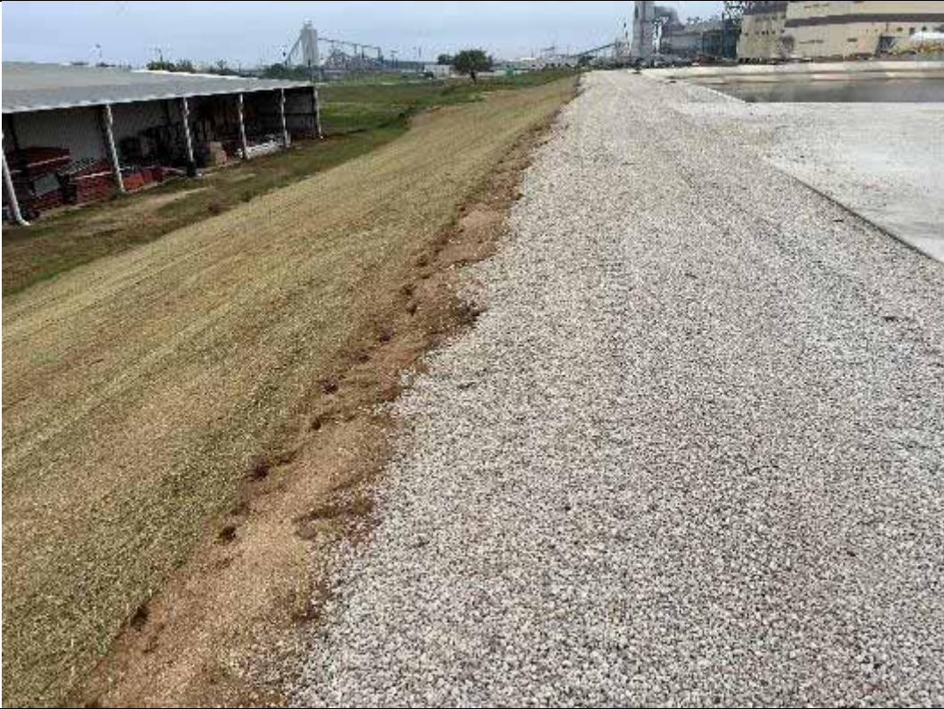
Photograph: 57 East Plant Drains Pond – standing on the northwest corner – facing south. Photo taken 11/16/2023.
