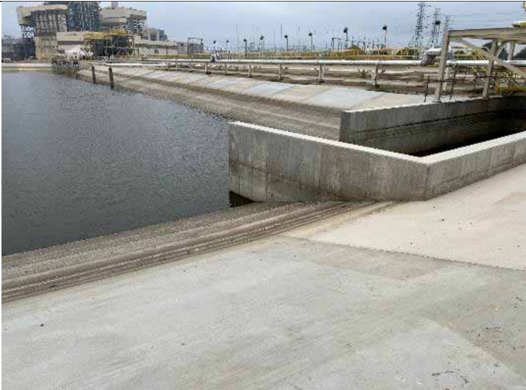
Photograph: 56 East Plant Drains Pond – standing on the northwest corner – facing south. Photo taken 11/16/2023.
