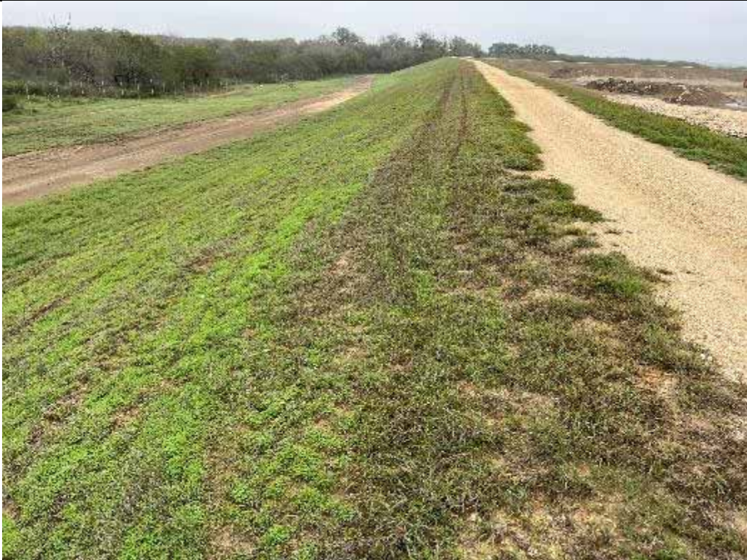
Photograph: 2 Fly Ash Landfill – standing on northwest corner – facing east. Photo taken 11/16/2023.
