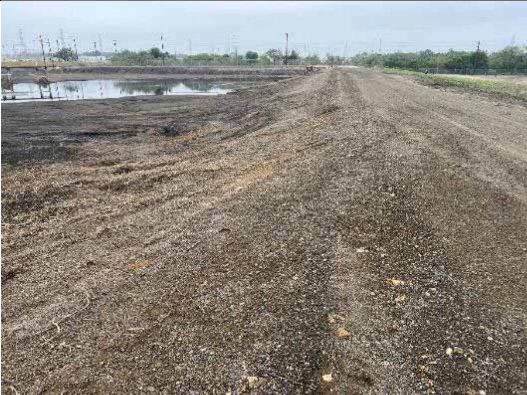
Photograph: 25 North Bottom Ash Pond – standing on southeast corner – facing north. Photo taken 11/16/2023.
