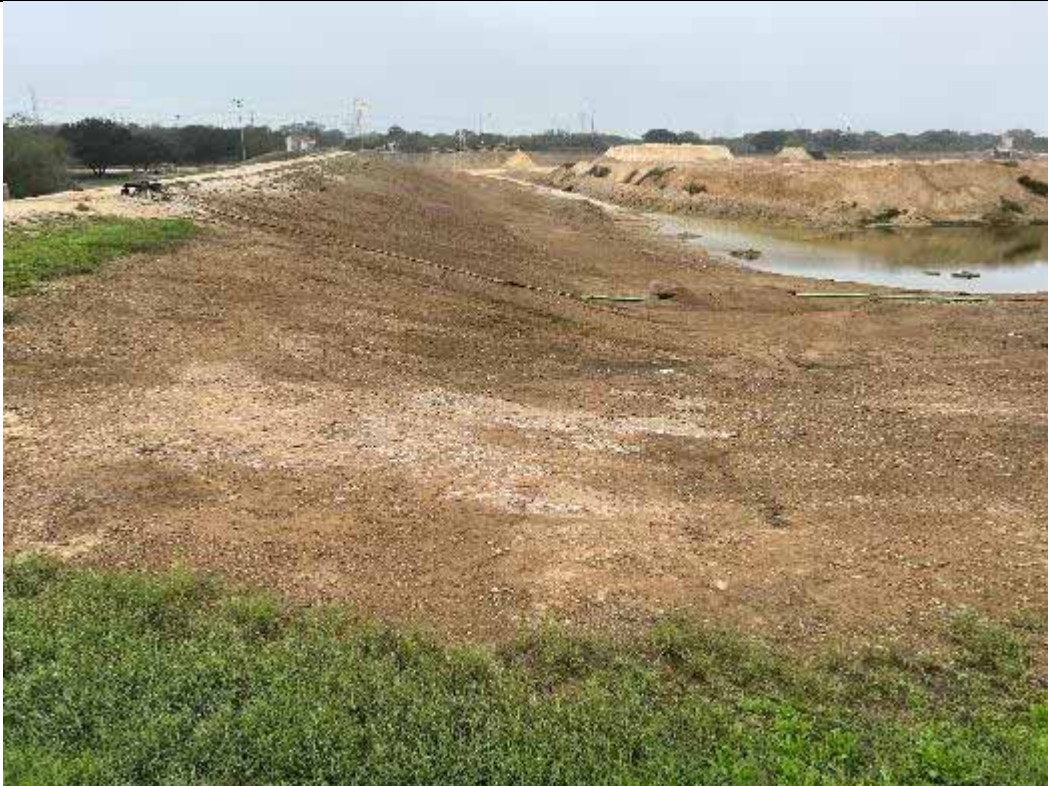
Photograph: 7 Fly Ash Landfill – standing on southeast corner – facing west. Radial stacker located in southwest corner and stormwater discharge piping in southeast corner of landfill. Photo taken 11/16/2023.
