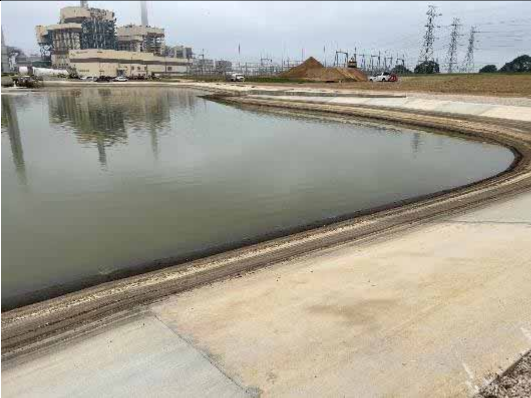
Photograph: 47 West Plant Drains Pond – standing on the northeast corner – facing southwest. Photo taken 11/16/2023.
