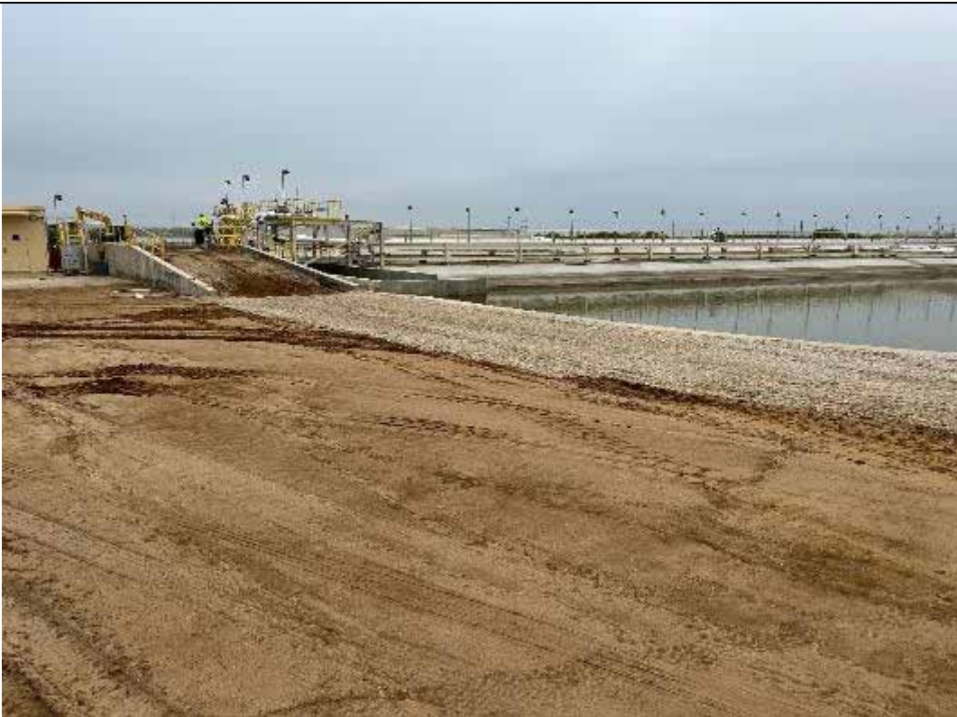
Photograph: 44 West Plant Drains Pond – standing on the northwest corner – facing southeast. Photo taken 11/16/2023.
