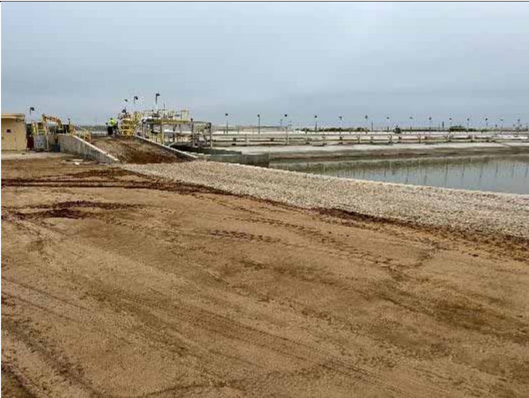
Photograph: 48 West Plant Drains Pond – standing on the northeast corner – facing south. Photo taken 11/16/2023.
