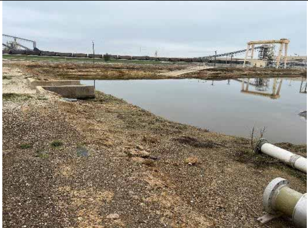
Photograph: 36 South SRH Pond – standing on the northeast corner facing southwest – spillway structure. Photo taken 11/16/2023.
