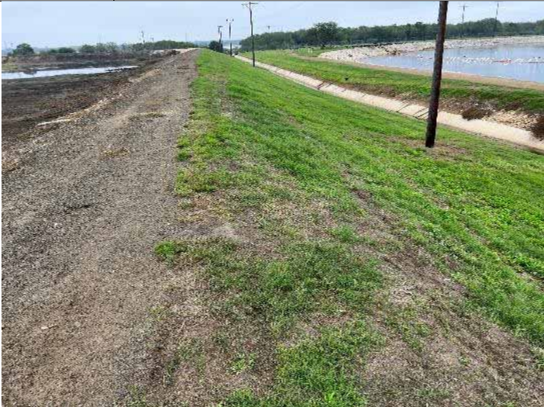
Photograph: 30 South Bottom Ash Pond – standing on southwest corner – facing east. Photo taken 11/16/2023.
