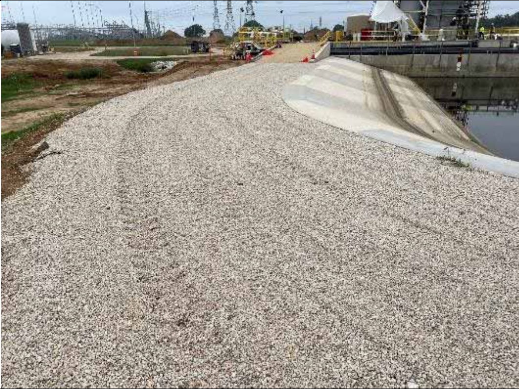
Photograph: 61 East Plant Drains Pond – standing on the southeast corner – facing west. Photo taken 11/16/2023.
