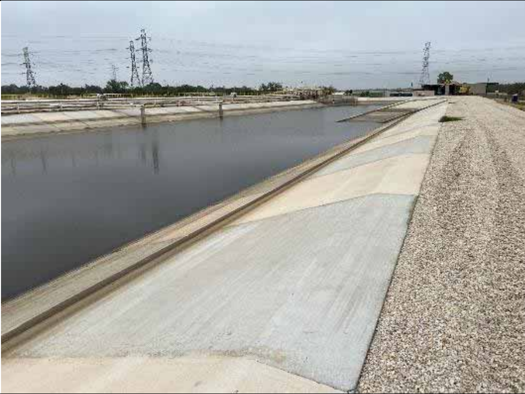
Photograph: 59 East Plant Drains Pond – standing on the southeast corner – facing north. Photo taken 11/16/2023.
