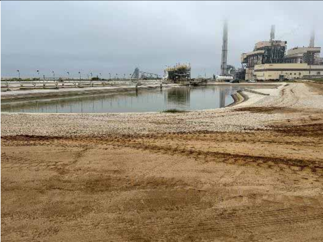
Photograph: 43 West Plant Drains Pond – standing on the northwest corner – facing south. Photo taken 11/16/2023.
