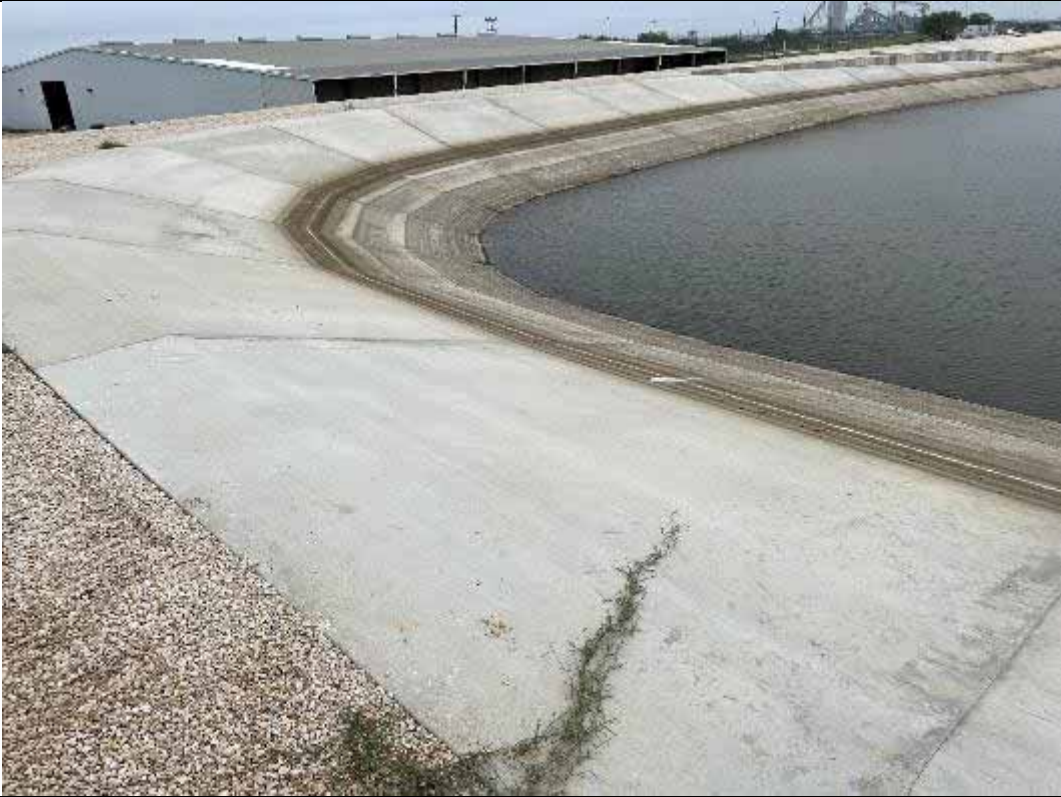
Photograph: 55 East Plant Drains Pond – standing on the northeast corner – facing southeast. Photo taken 11/16/2023.
