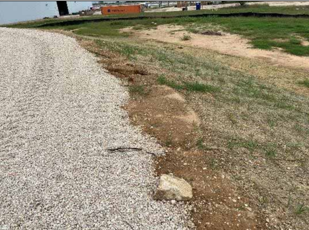
Photograph: 58 East Plant Drains Pond – standing on the southeast corner – facing east. Photo taken 11/16/2023.
