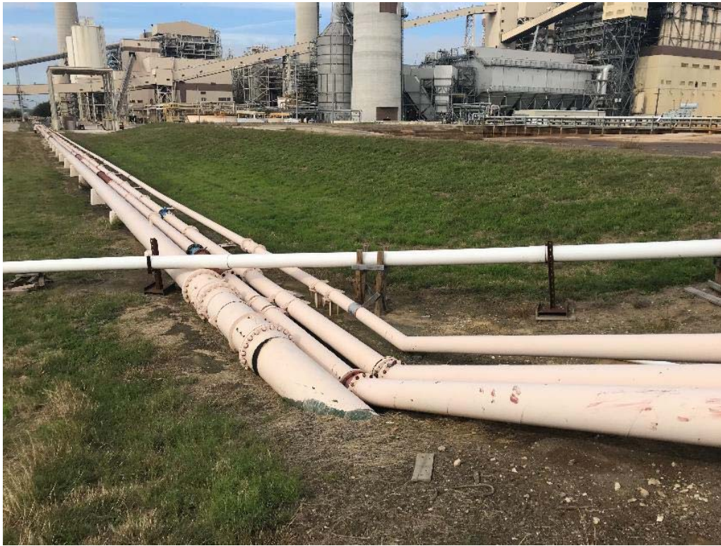
Photograph: 35 South SRH Pond – standing outside the southeast corner – facing northwest. Photo taken 12/18/18.
