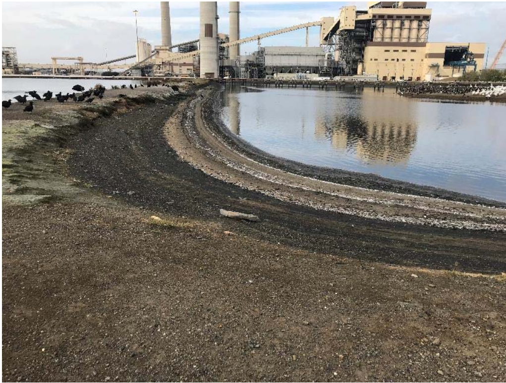
Photograph: 19 North Bottom Ash Pond – standing on southeast corner – facing west. Photo taken 12/18/18.
