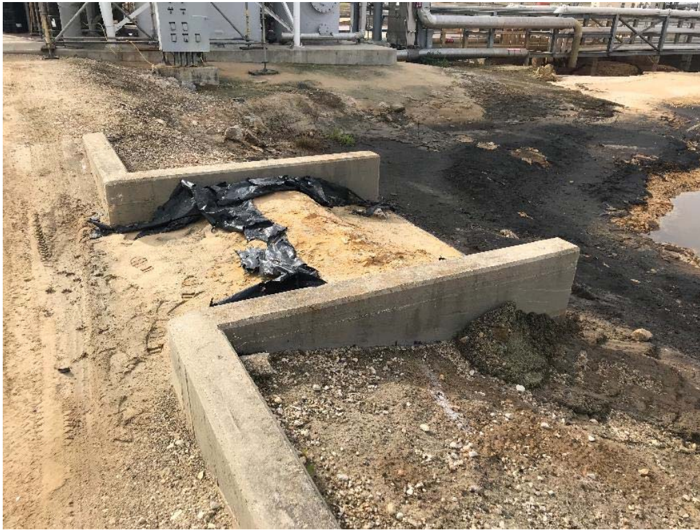
Photograph: 31 North SRH Pond – standing on eastern berm – facing southwest. Spillway structure. Photo taken 12/18/18.
