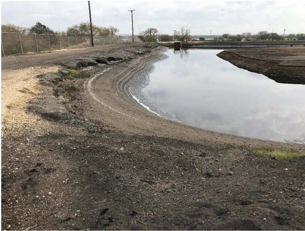
Photograph: 17 North Bottom Ash Pond – standing on northwest corner – facing east. Photo taken 12/18/18.
