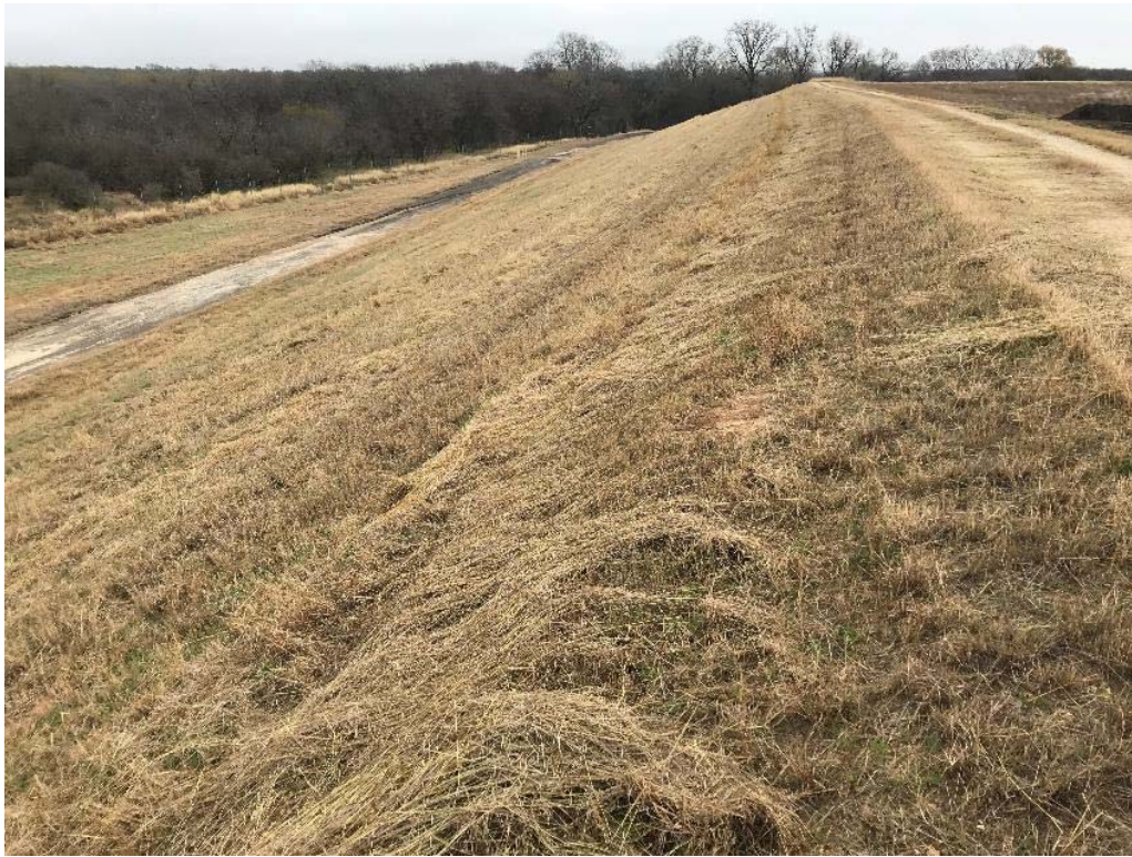
Photograph: 5 Fly Ash Landfill – standing on northern berm – facing east. Photo taken 12/18/18.
