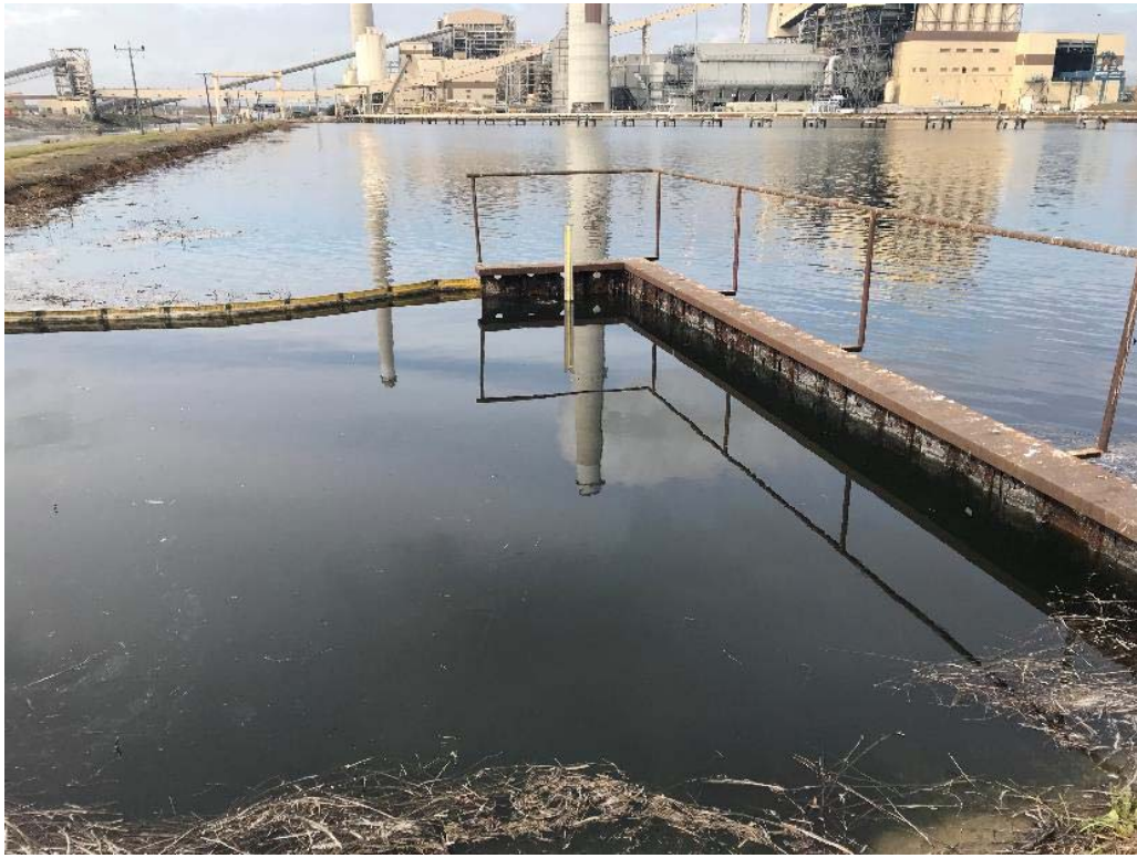
Photograph: 25 South Bottom Ash Pond – standing on southeast corner – facing west. Outfall intake noted below water level. Photo taken 12/18/18.
