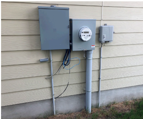
Underground Lines Connected to Electric Meter
