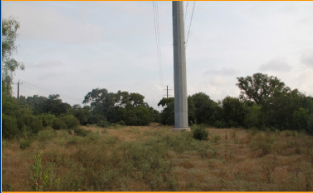
100ft clearing around transmission structure
