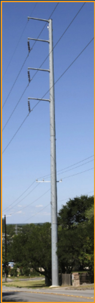
Single Circuit Structure
