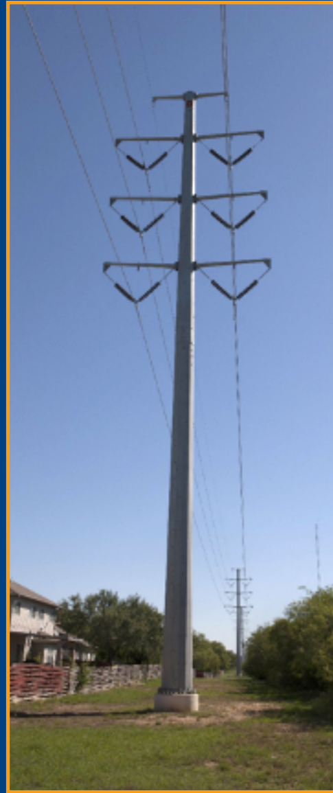
Double Circuit Structure
