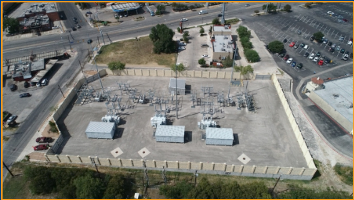
Exeter Substation – Typical Air Insulated Substation (AIS)
