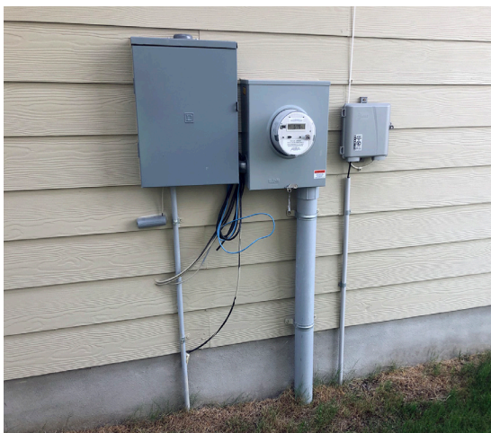
Underground Lines Connected to Electric Meter
