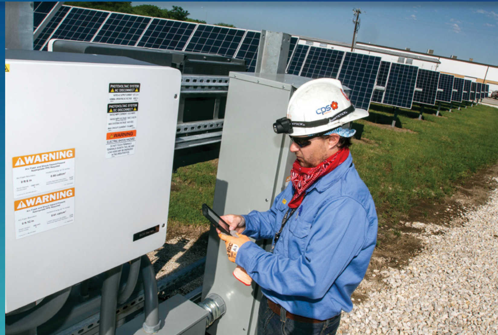
Eric Bosanko, Operator Control Room, reviews Solar + Battery Energy Storage system's data.
